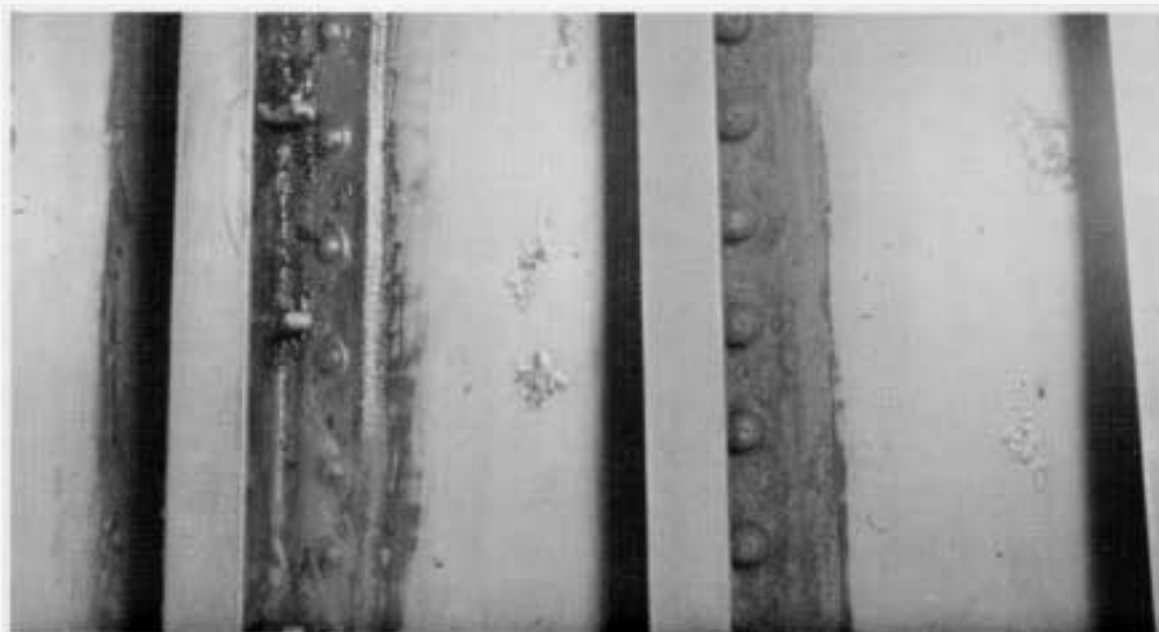
FIGURE 3. C-130 fuel tank after removal of the Buna-N shows the corrosion blisters and pockets.
